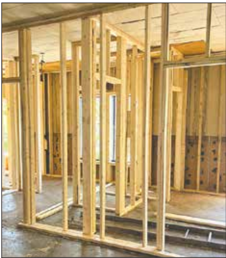
Upstairs the former billiards hall is being outfitted as four short term rental apartments.
