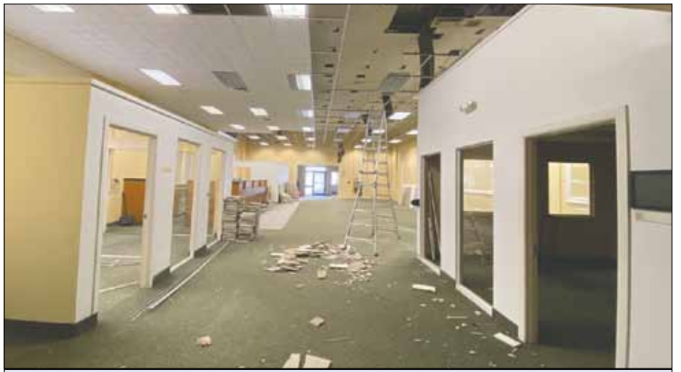
Before! — Prior to renovations , architectural elements of the historic First National Bank on Glen Street — familiarly known at "The White Bank" — were largely hidden behind drop ceilings and modern offices. View is looking west, from the back wall of the now-Worksmart shared office space toward the front door onto Glen Street. Photo provided
